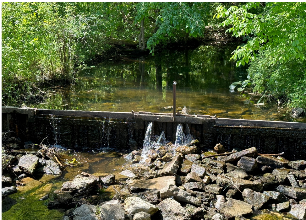
Current Structure - Holes in Metal
