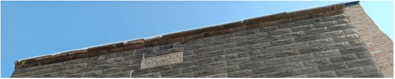
Photo 9: Cornice along top of south wall is broken.
