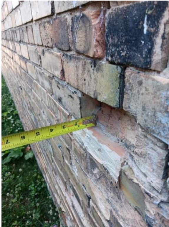
Photo 3: Missing brick along west side of building.
