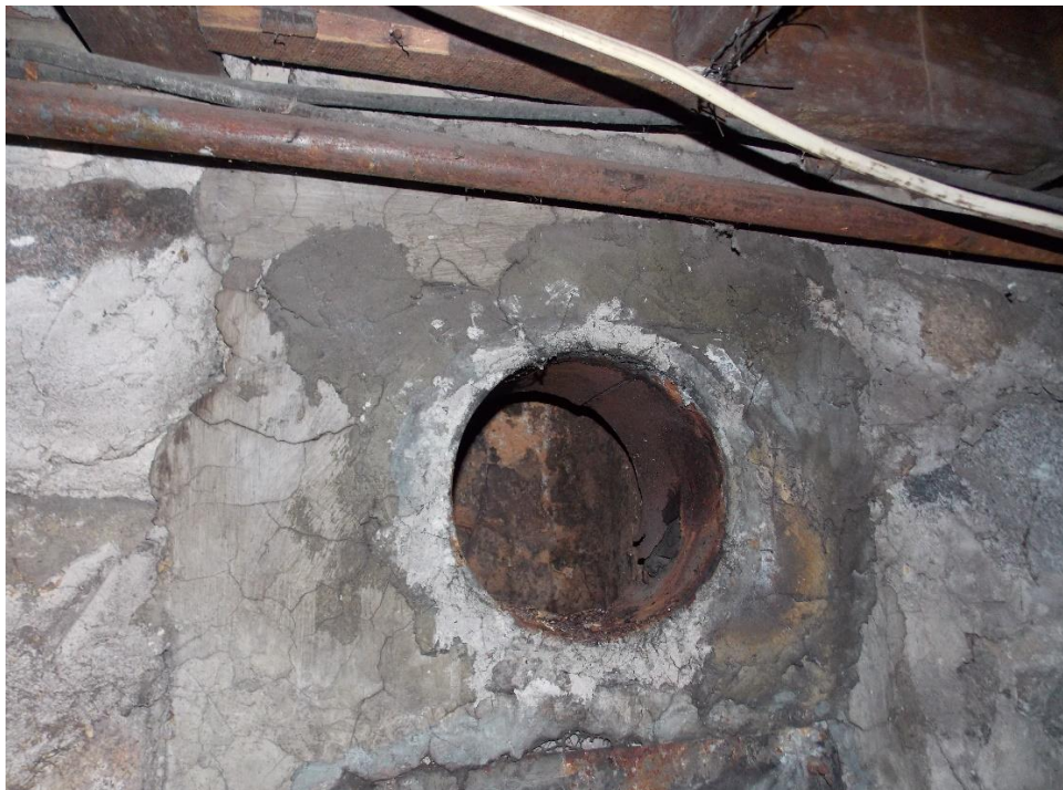
HA-26: Penetration Flue Insulation
