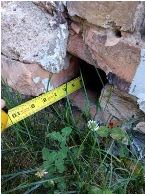
Photo 4: Missing brick along west side of building.
