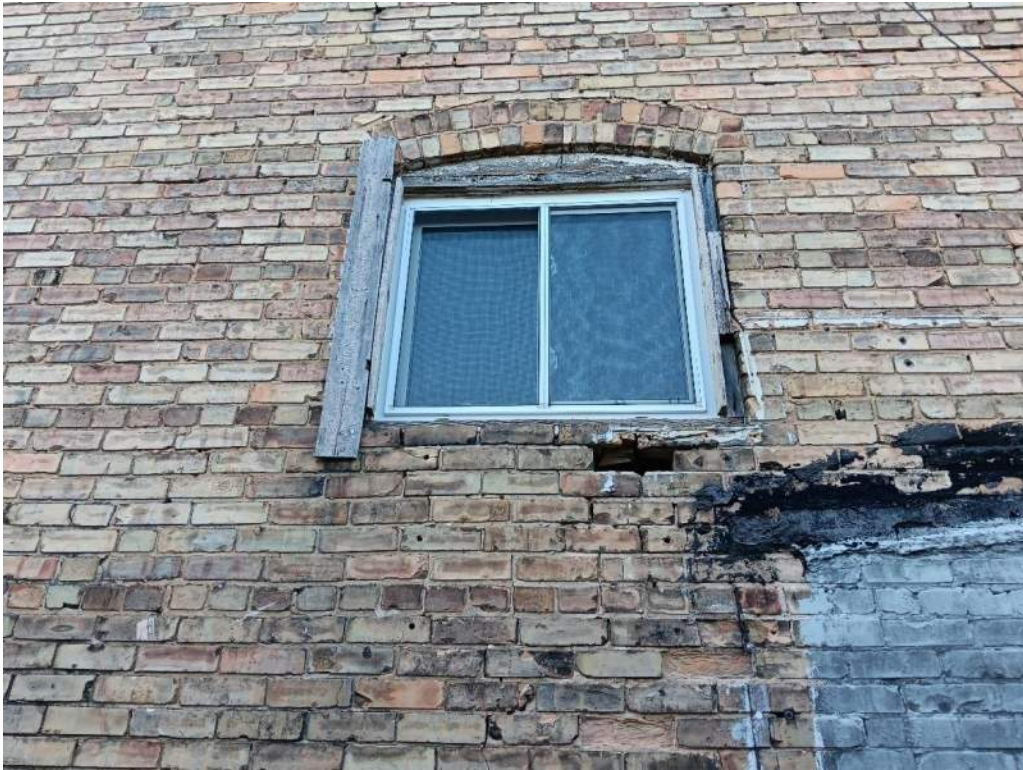
Photo 5: Missing brick around window on west side of building.
