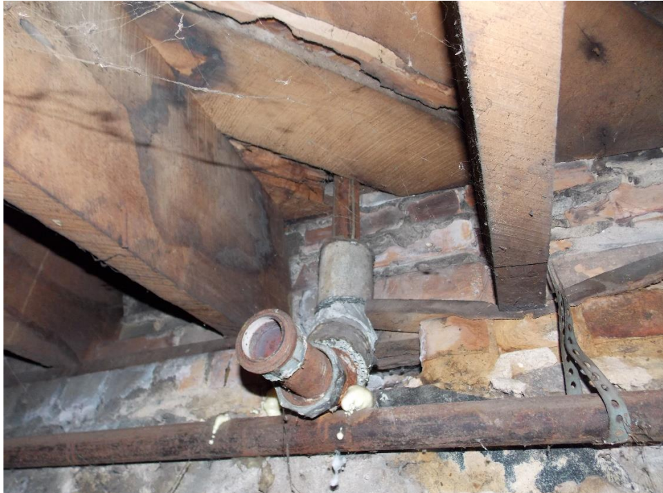
HA-25: Aircell Pipe Insulation
