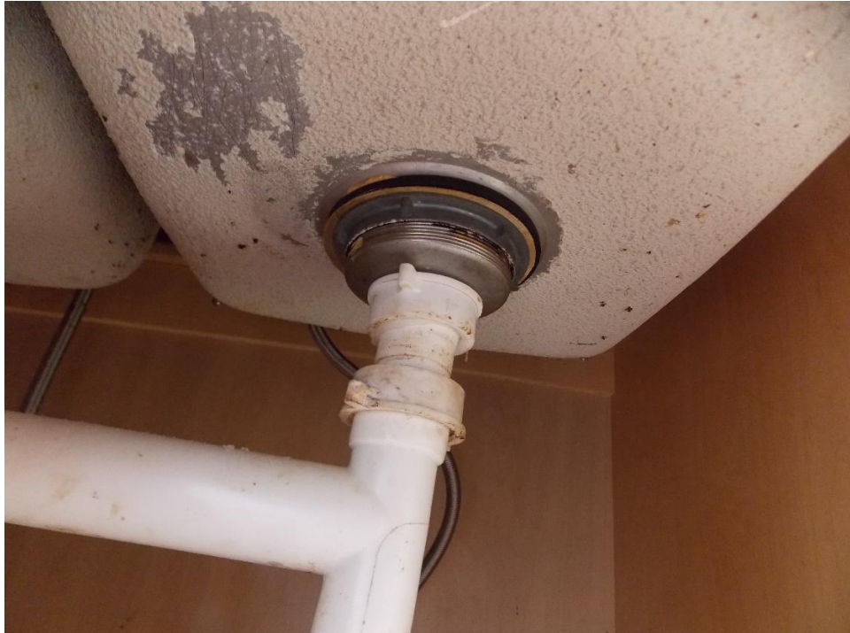
HA-39: White Sink Undercoat
