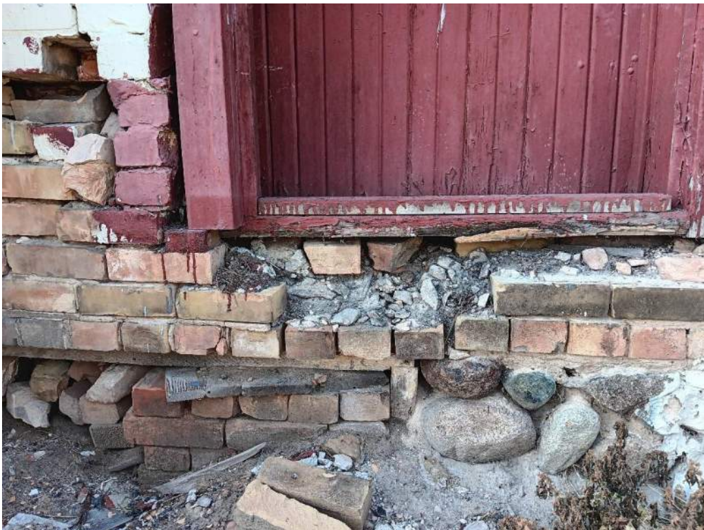
Photo 6: Missing and loose bricks on north side of building.
